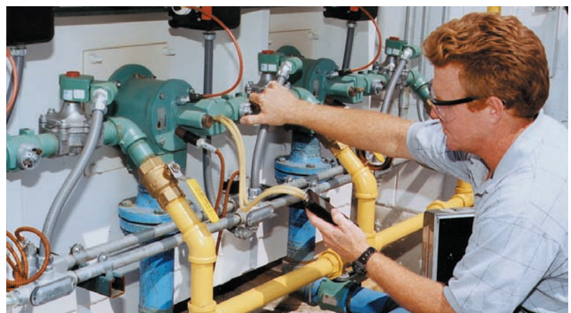
A burner technician can show you where to measure air pressure. Check the pressure inputs on your burner monthly.
